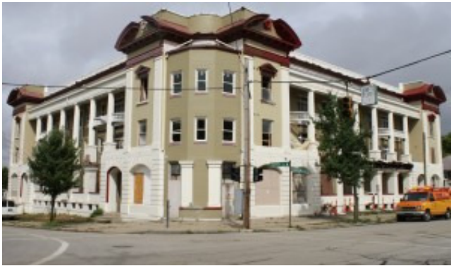
The reconstruction of the Elberon building at the corner of West Eighth Street and Elberon Avenue is moving along as scheduled. The exterior, though still not completed, is already a vast improvement from how the building looked prior to construction starting. Kurt Backscheider/Staff
