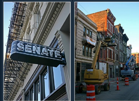
Work nears completion on Model Group's Trinity Flats Infill and restoration project near 14th & Vine streets [TOP]. Senate, a new gastropub, is scheduled to open soon near 13th & Vine streets [LEFT], while work begins in earnest on the latest phase of the Gateway Quarter which will include new apartments and businesses [RIGHT].
